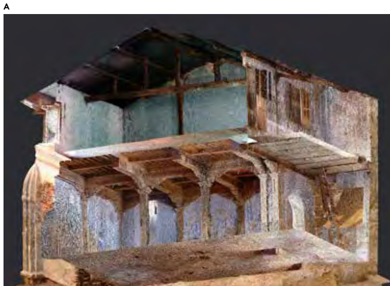
A Sectional view of the dense point cloud model of Tankshal ni Pol Mosque depicting wooden structural system. Image: Zeus Pithawalla (Center for Heritage Conservation, CEPT Research and Development Foundation, Ahmedabad) based on 3D LiDAR scanned data obtained by a surveying agency Shayona Management Services Pvt. Ltd. (March 2021)
